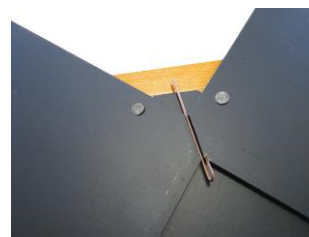
Nailing in the batten and fixing the disc rivet in the joint between 2 slates
