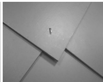
Placing of the next slate over the disc rivet and bending of the disc rivet, not too strong so that movement of the slate is still possible
